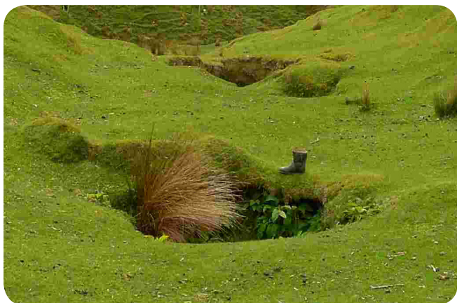
Holes created by partial collapses of a tunnel gully in the Tararua District.
