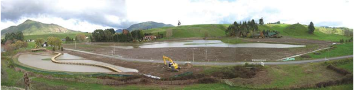
Figure 5. Wetland at Lake Okaro, Rotorua, New Zealand during construction (below) and once vegetated (over page).
