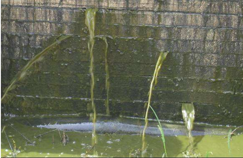
Photo 10. Liquid FDE flowing through the wooden slatted 'weeping' wall.
