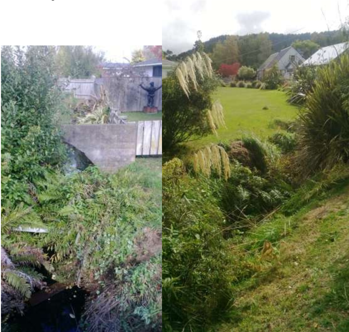
Photos 12 & 13: Restriction to flow caused by small channel, vegetation and access structure downstream of 22 Lee Street. Photo on right is immediately downstream.
