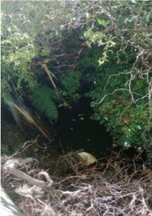
Photo 11: Another congested reach in Miro Street Drain.
