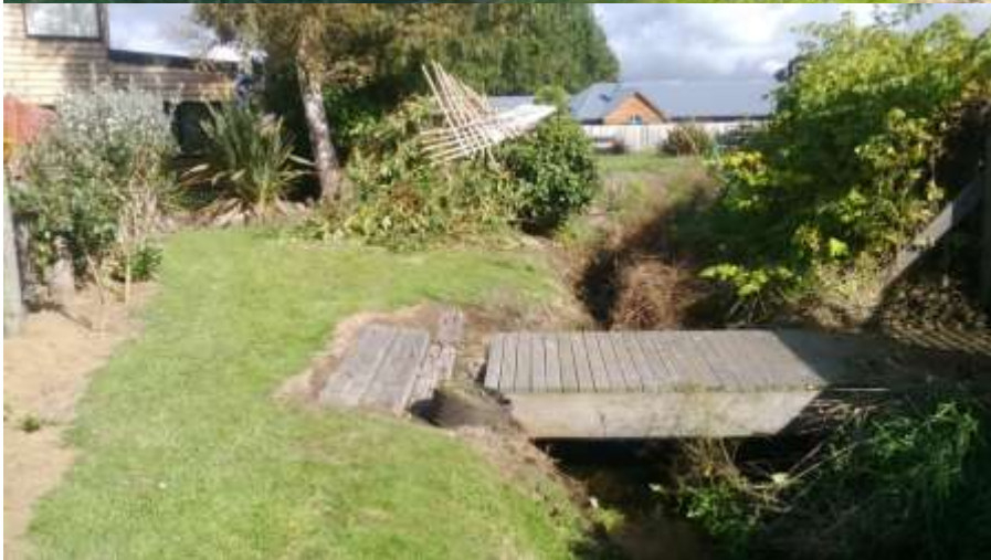
Photos 18 & 19: Obstructions to flow outside 105 Miro Street - Retaining wall for plant, footbridge and 1.5m high green waste pile.
