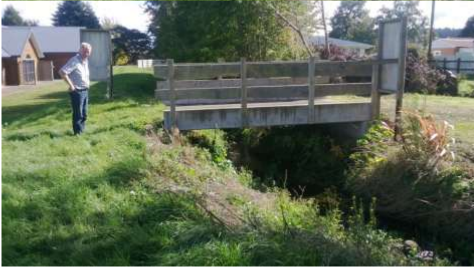
Photos 23 & 24: Miro Street Drain Stopbank looking towards Mangawhero Terrace. Note unconsented bridge access to 1A Martin Place.
