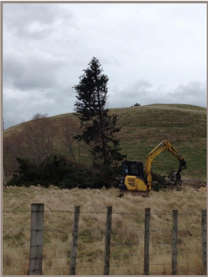
Photo 10: Contractors using digger to control large contorta trees adjacent to SH1, (M. Matthewson).
