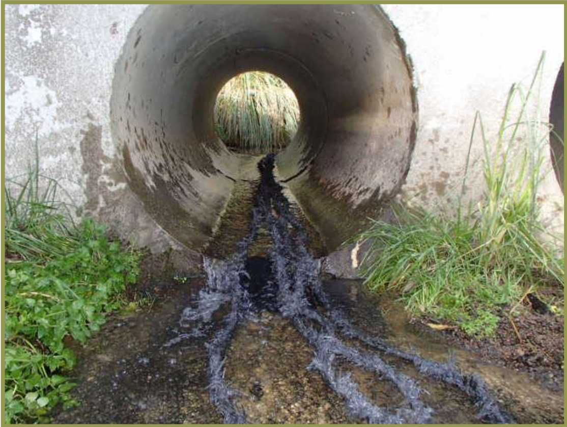
Photo 6: One of the fish pass solutions using mussel rope through a perched culvert in Koputaroa catchment.
