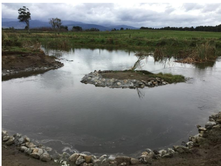
Photo 4 The fish pass on the Hokio Stream weir was commissioned on 5 May. The weir is submerged in this photo but is situated from the small island in the centre of the photo out to the far bank of the Hokio Stream. The fish pass is the rock lined loop in the foreground. This has a very low gradient that will allow all fish species to access the lake.
