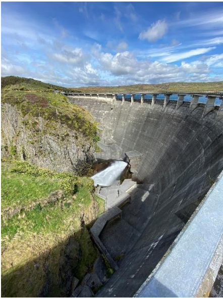
Figure 9. Maowhango Dam Disperser Valve.
