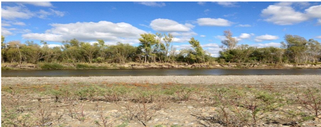
Photograph 2: Erosion on left bank at McDonald river distance 14.6 km
