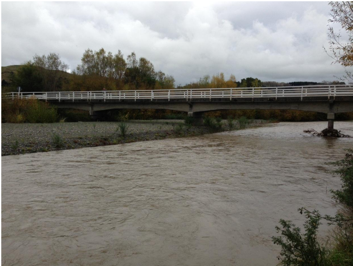
Photograph 8: Significant aggradation at Coulters Line Bridge 25.9 km
