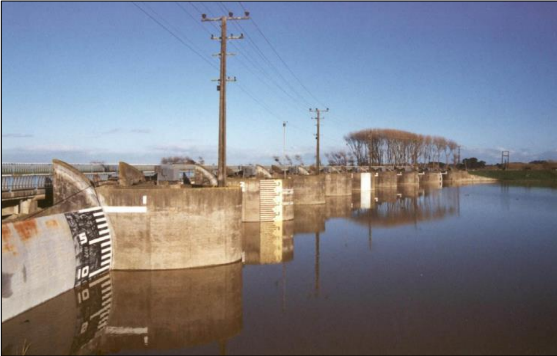
Figure 2-1 Moutoa Sluice Gates during high flows. The white dash against Gate 1 indicates the maximum design water level of 8.25 m MSL (7.85 m NZVD16). Source 'Moutoa Sluice Gate & Floodway – Helping keep our Region safe'
