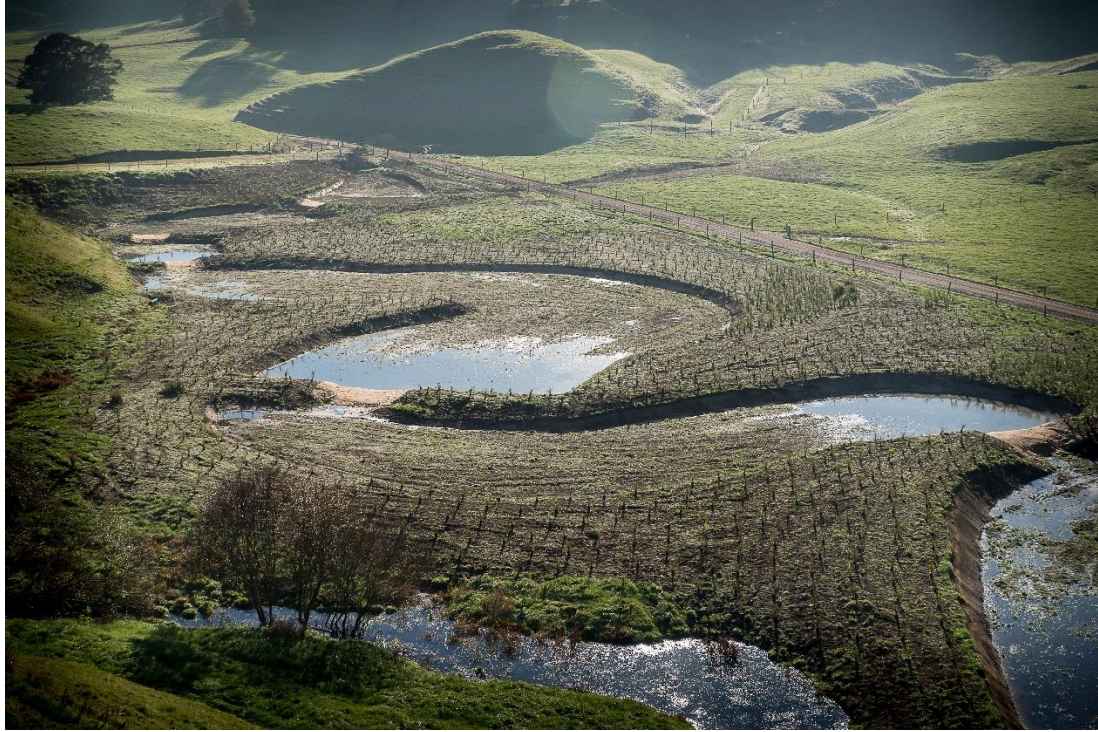
Figure 1: Constructed treatment wetland at Putaruru showing shallow, flat-bottomed wetland bays before the wetland has been planted.
