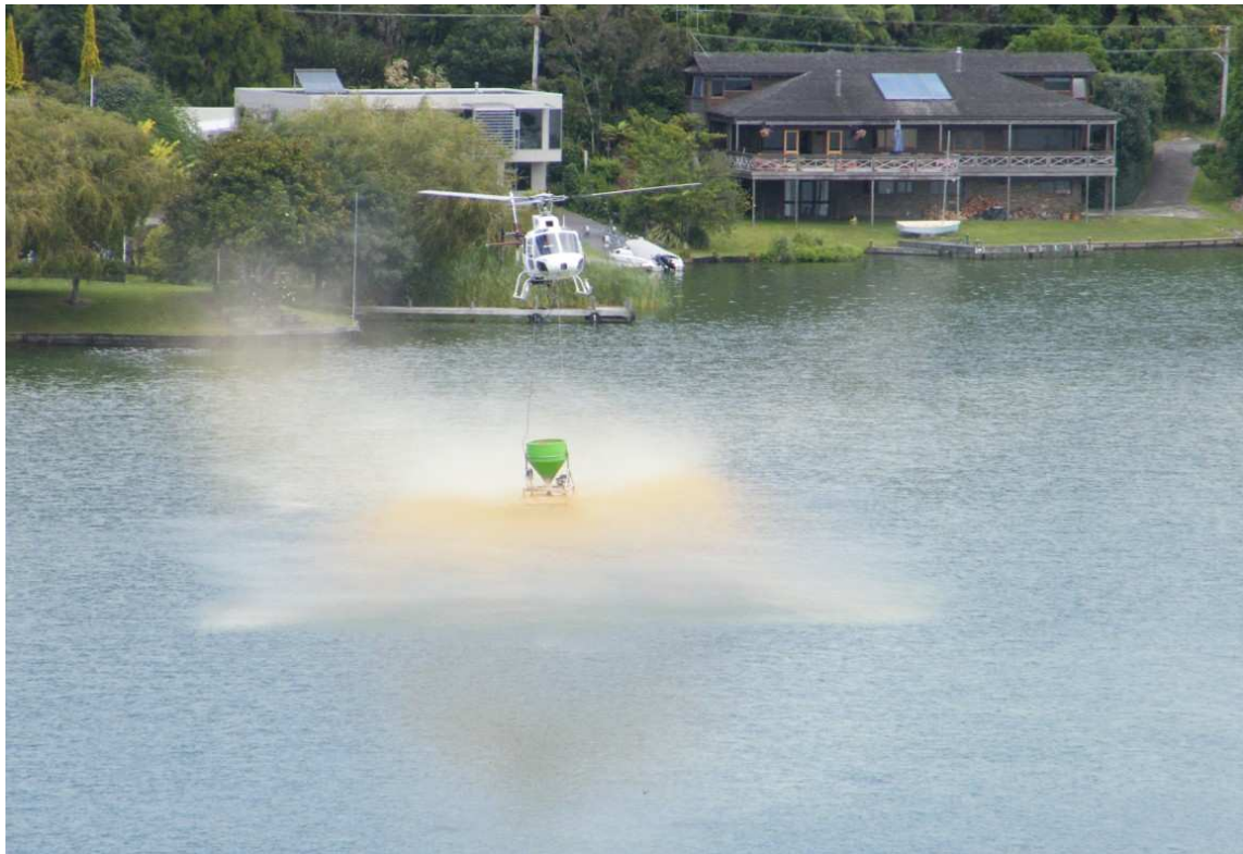
Figure 48. Application of Aqual P TM as a slurry from a helicopter on Okawa Bay, Lake Rotoiti. The helicopter position was controlled using GPS navigation. [Photo: Graham Timpany, NIWA, Rotorua].
