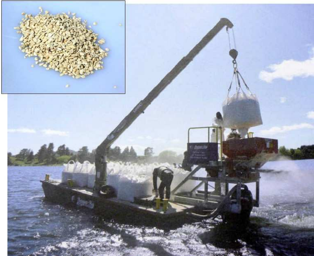
Figure 49. Application of coarse granular Aqual P™ on Lake Okaro in September 2007, using a fertilizer spreader on a barge. The product being applied is shown in the inset.
