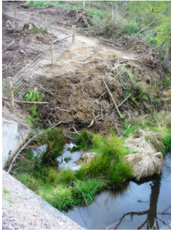
Figure 1: Poor operational practice in clearing fence line in riparian area
