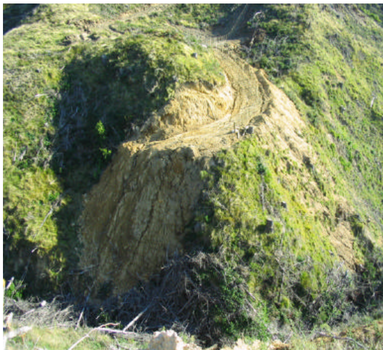
Figure 4: Fence line construction and soil disposal directly into a watercourse in association with forest to farm conversion
