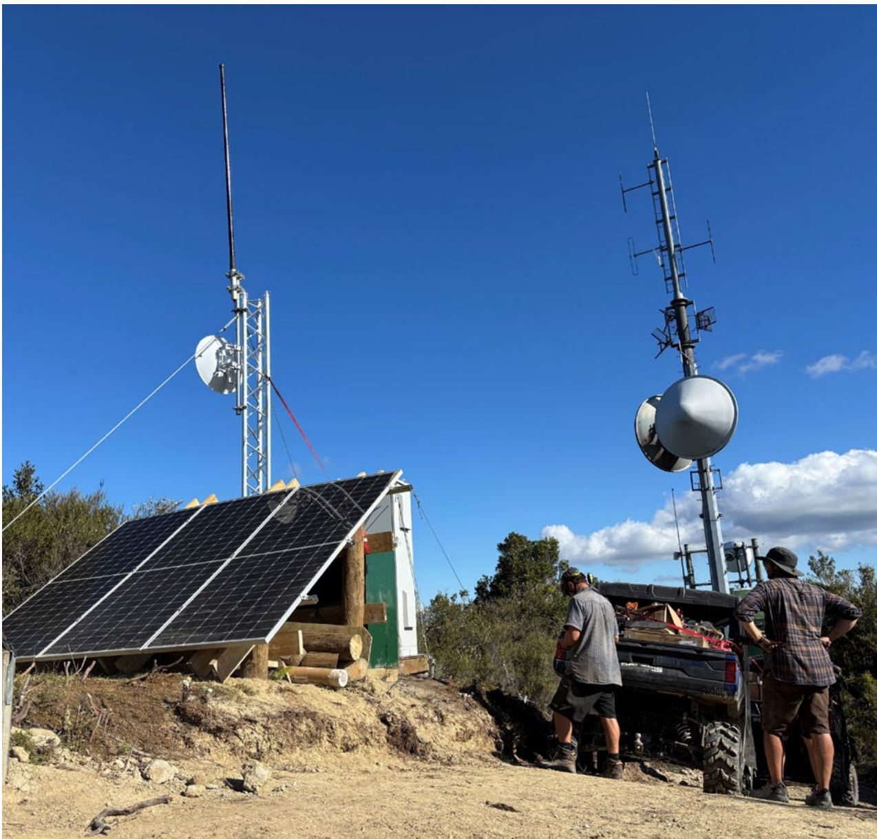
Installing environmental data monitoring equipment
