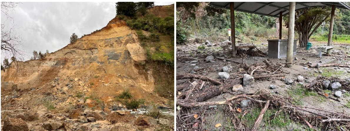
Figure 2: (Left) Land slip July 2026 and (right) BBQ Rockfall inundation July 2026
