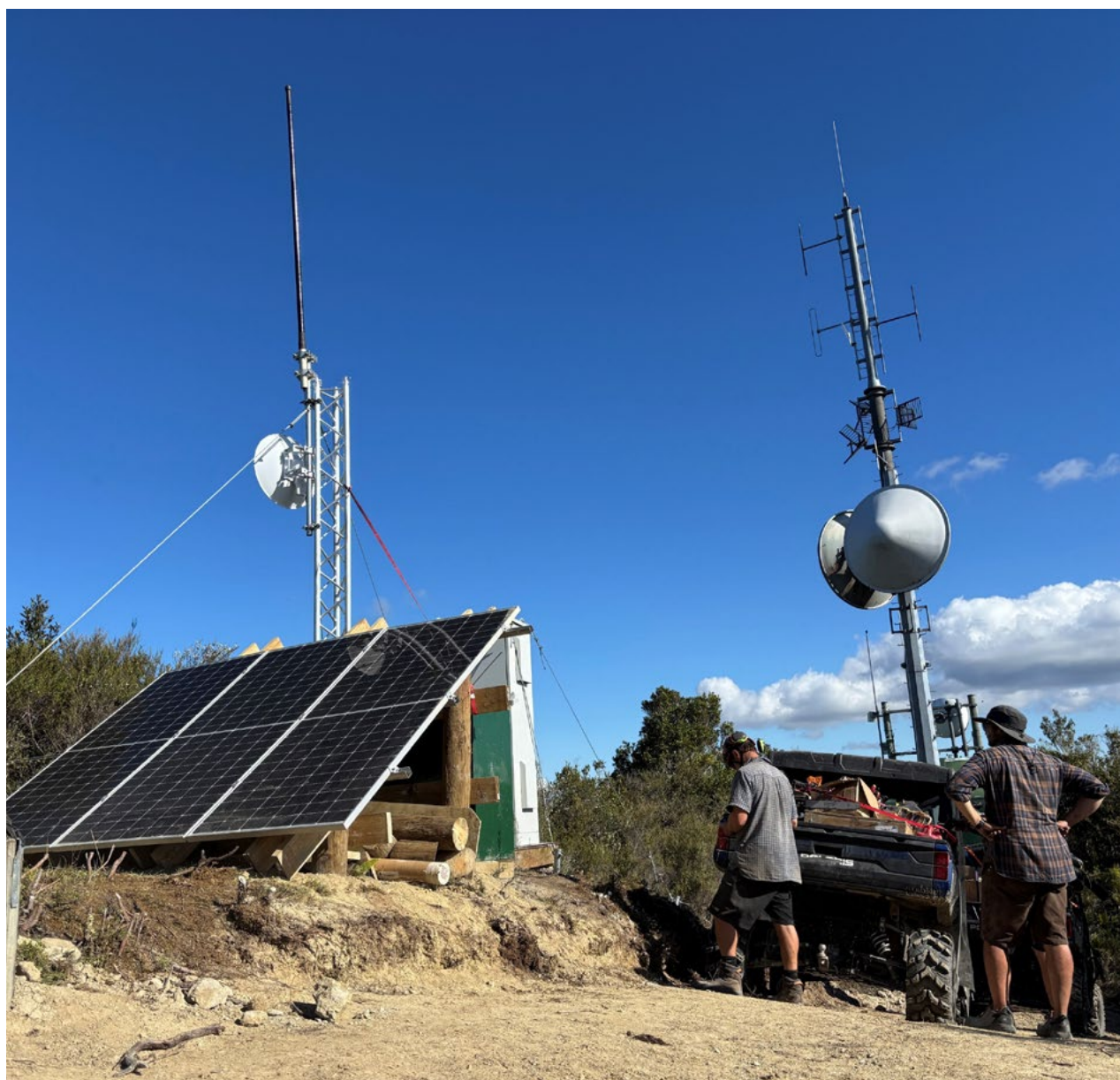
Installing environmental data monitoring equipment
