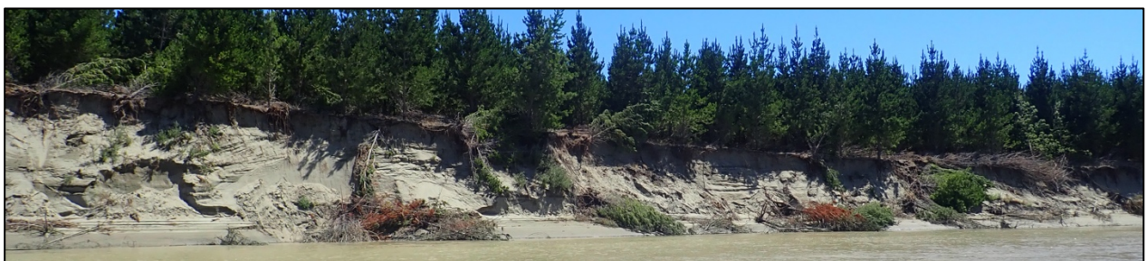
Eroding channel margin adjacent to plantation pine forest opposite Fernbird Flat.
