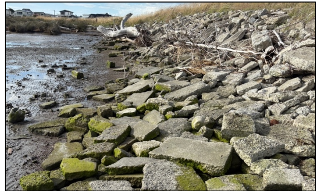
Sparse cover of Ulva spp. on rip-rap rock armouring.
