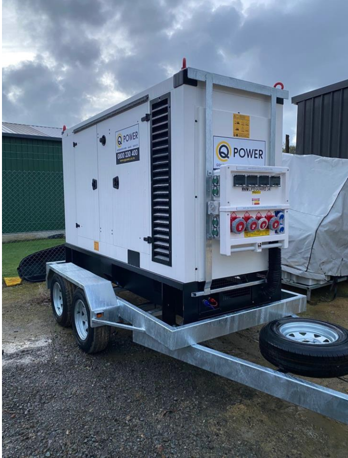
New 250KVA Generator
