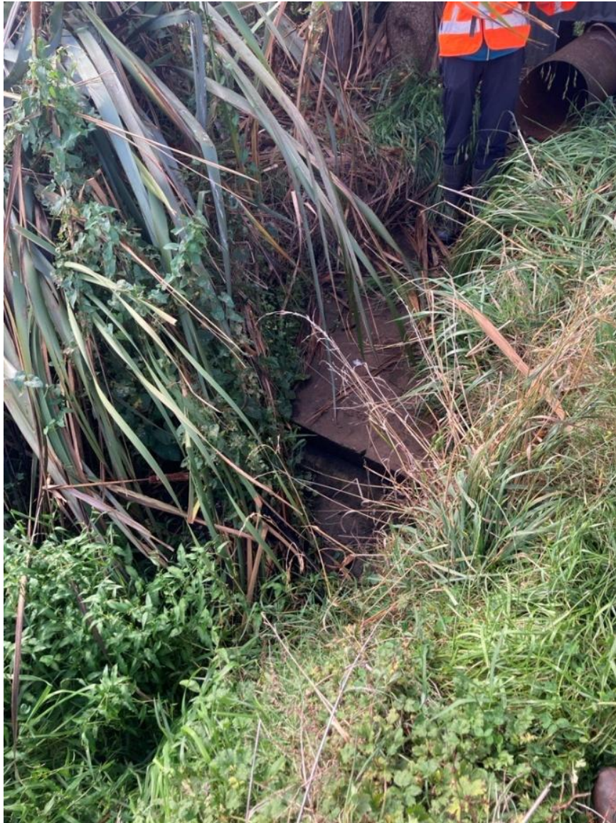
Figure 17: Pumphouse outflow on Pukepuke Lagoon on 13/4/2026
