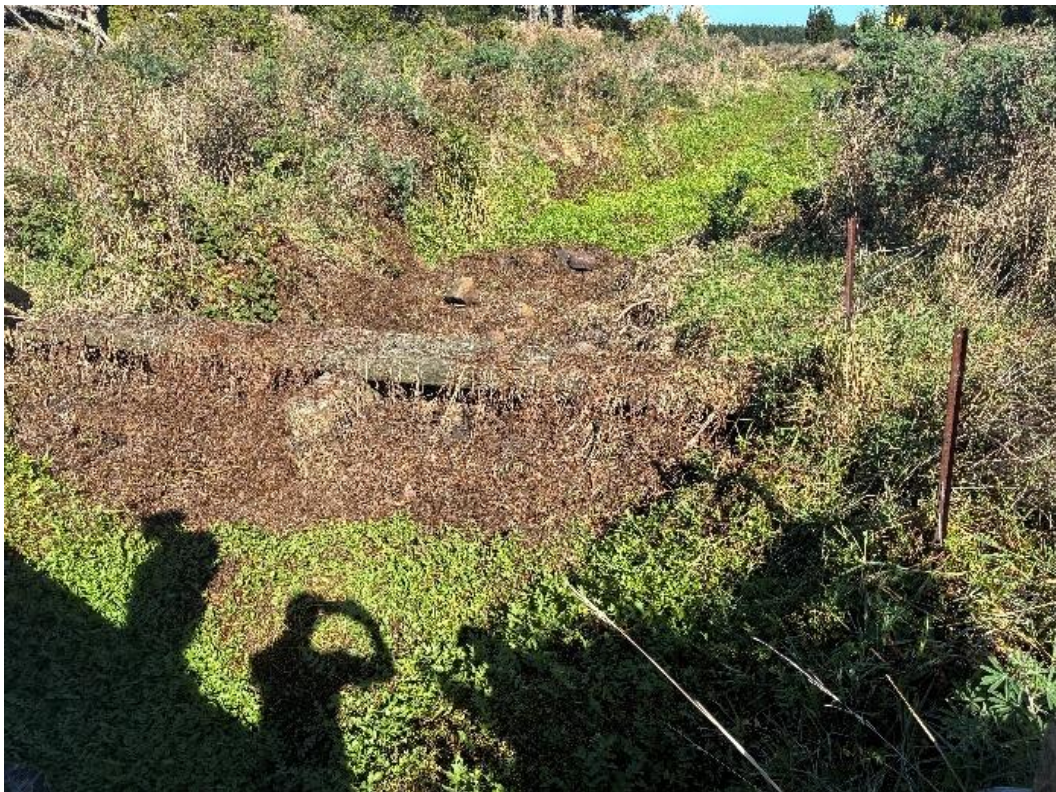
Figure 29: Overgrown weir at north-west boundary of Pukepuke lagoon
