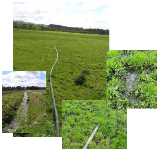
Effluent discharge to land system
