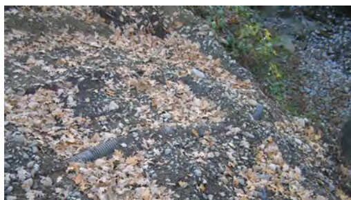
Nova Flow pipe running beneath the yards, and exiting directly over Porewa Stream.
